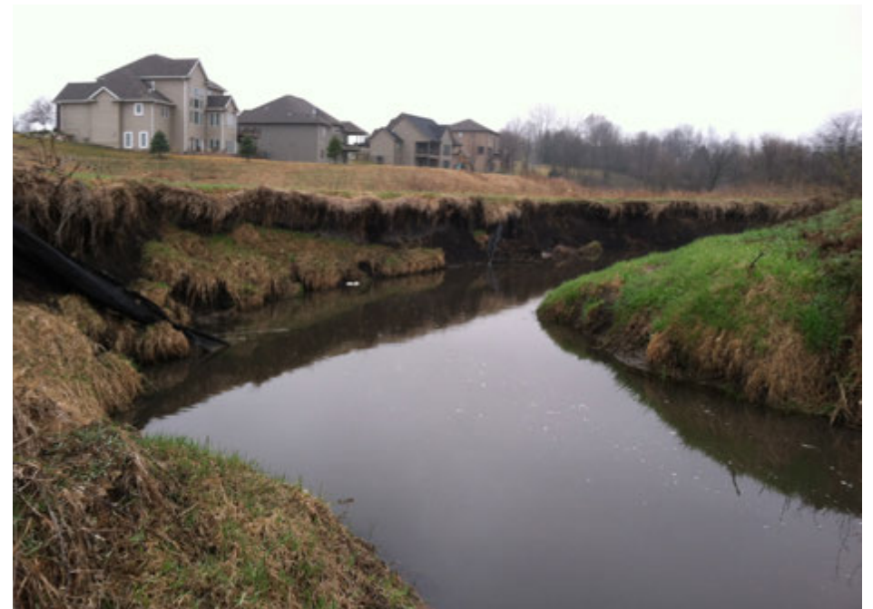
UNSTABLE: Rapid erosion occurring along Upper Walnut Creek.
