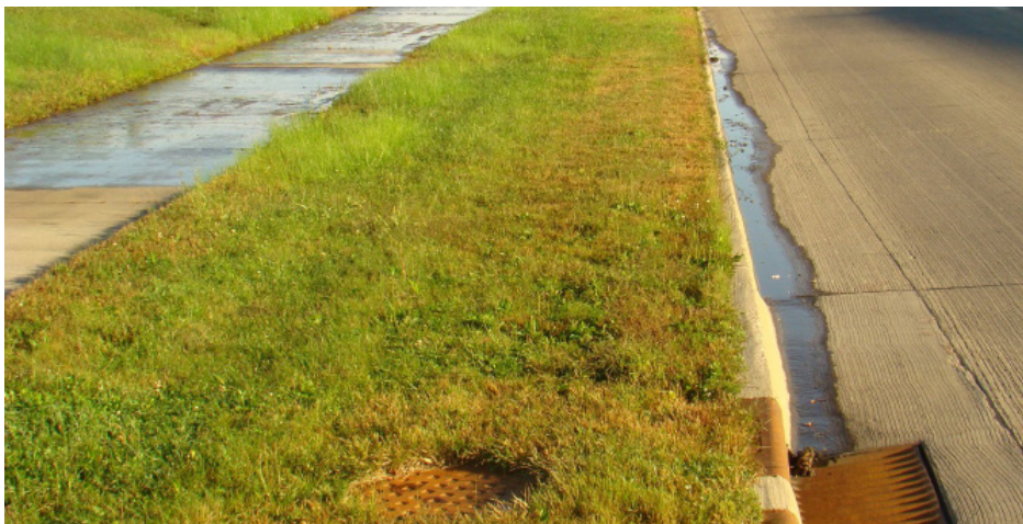
Because of soil compaction, moisture is unable to percolate through the soil. Here it is forced to seep across the sidewalk and over the curb because it cannot penetrate subsoil layers.
